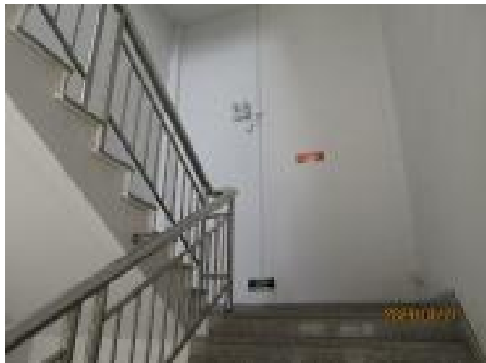
Emergency Light in the Staircase.jpg
