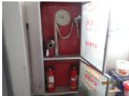
Fire Hydrant and Fire Extinguishers.jpg
