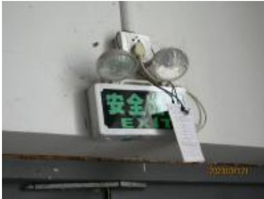
Emergency Light and Exit Sign.jpg
